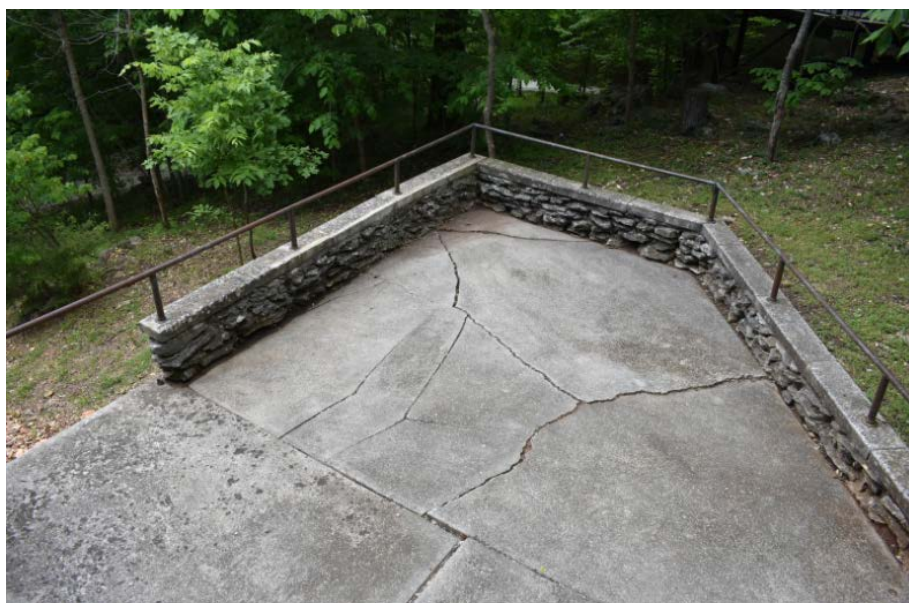
Figure 25: Partial View of the Landing (c. 1960), Contributing Structure. Image taken by Michelle Diedrich, Spring 2017.
